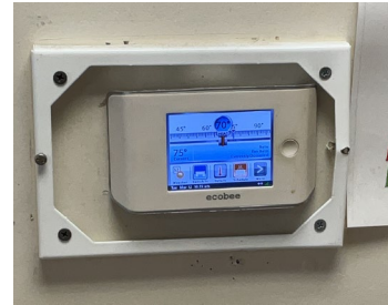
Ecobee Wi-Fi Thermostat Room E9
