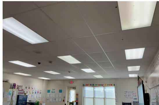
T8 Fluorescent Lighting – Classroom E6
