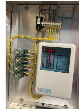
Paragon Time Clock Control Room
