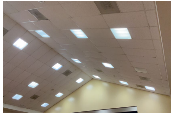
T8 Fluorescent Lighting – PE Room
