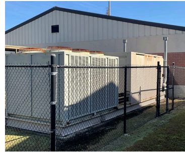
Outside Air Unit (1 of 2)
