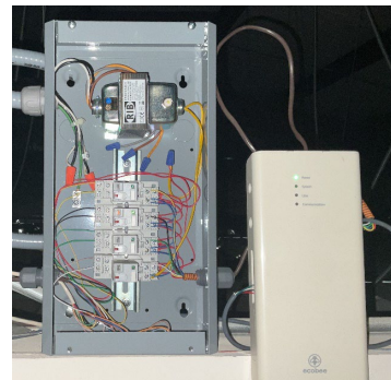
Ecobee Central Control Panel Attic
